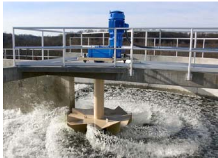
Oxidation ditch with Mechanical Aerators
